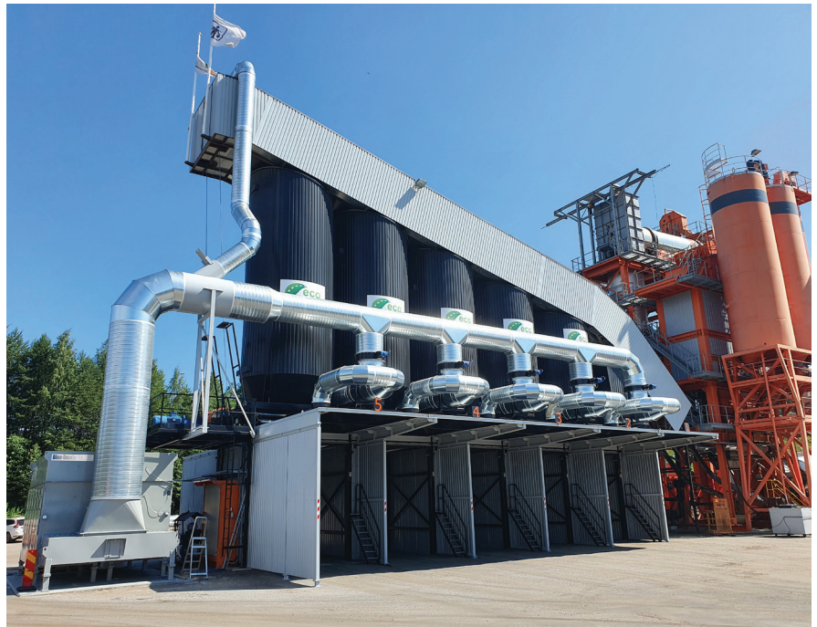
This picture shows the Blue Smoke Control collector and ductwork along the silo loadout system at Peab Asphalt's Lahti asphalt plant. Photo credit: Julius Jäntti
