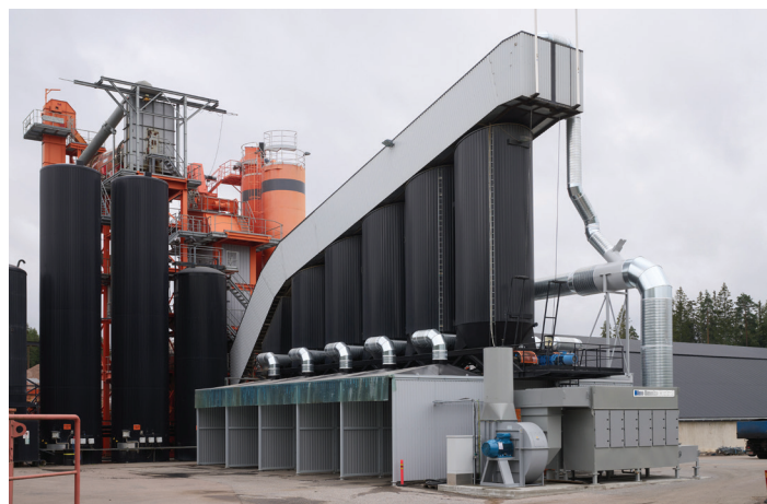
This side of the Blue Smoke Control collector system shows the collector fan that pulls fume into the filter system. Photo credit: Julius Jääntti
