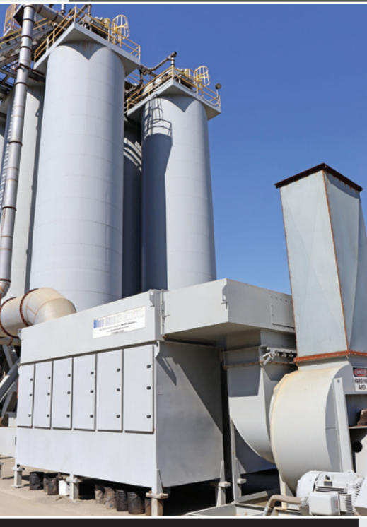
Above: Blue Smoke Control system from Butler-Justice, Inc. shown in operation at R.J. Noble Company in Corona.
